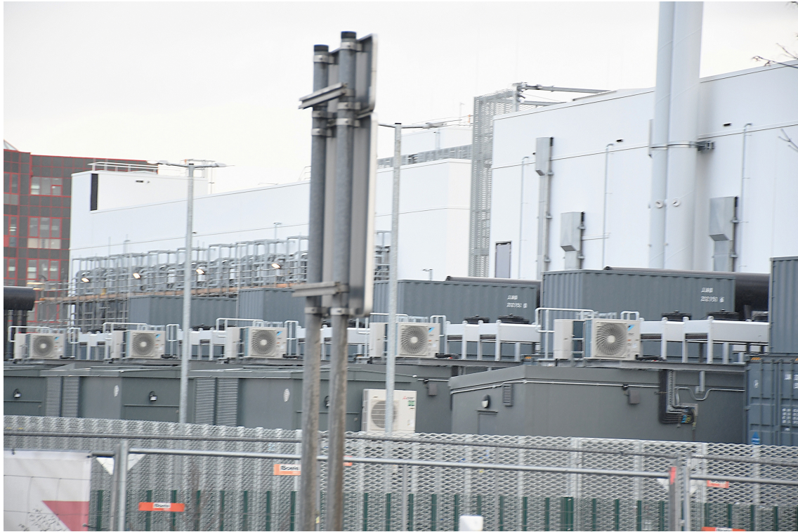
Figure 17: Lines of Air Conditioners and Cooling Towers behind a Data Center in Brandenburg Source: Image by the Authors
