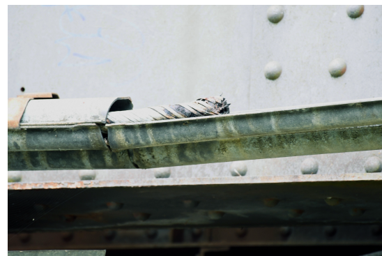
Figure 19: Broken Cable Source: Image by the Authors
