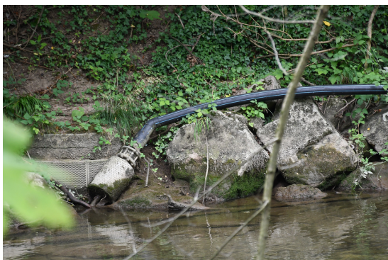
Figure 18: Unplugged Pipe Source: Image by the Authors
