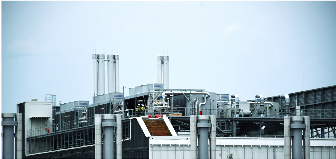
Figure 16: Cooling Towers over a Data Center in Frankfurt am Main
